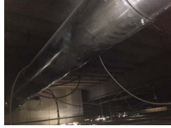
Fig. 6. Dropped Ceiling Ductwork
